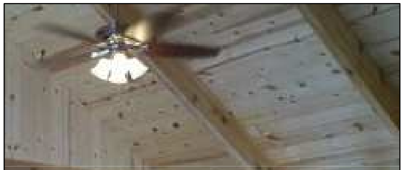
The Phase 2 ceiling finish knotty pine boards are installed over the 3x12 rafters included in the Phase 1 log shell kit
